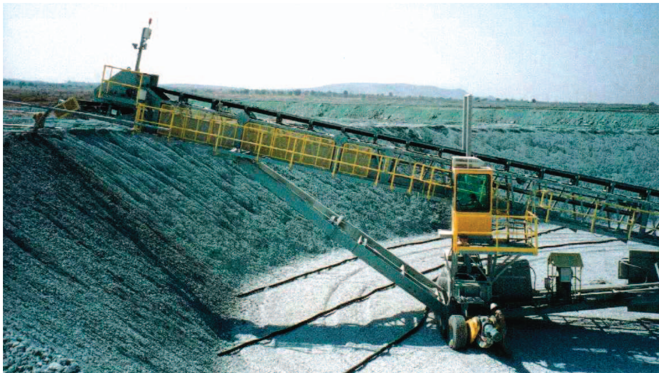
Heap leach material being placed on a pad using a radial stacker.
