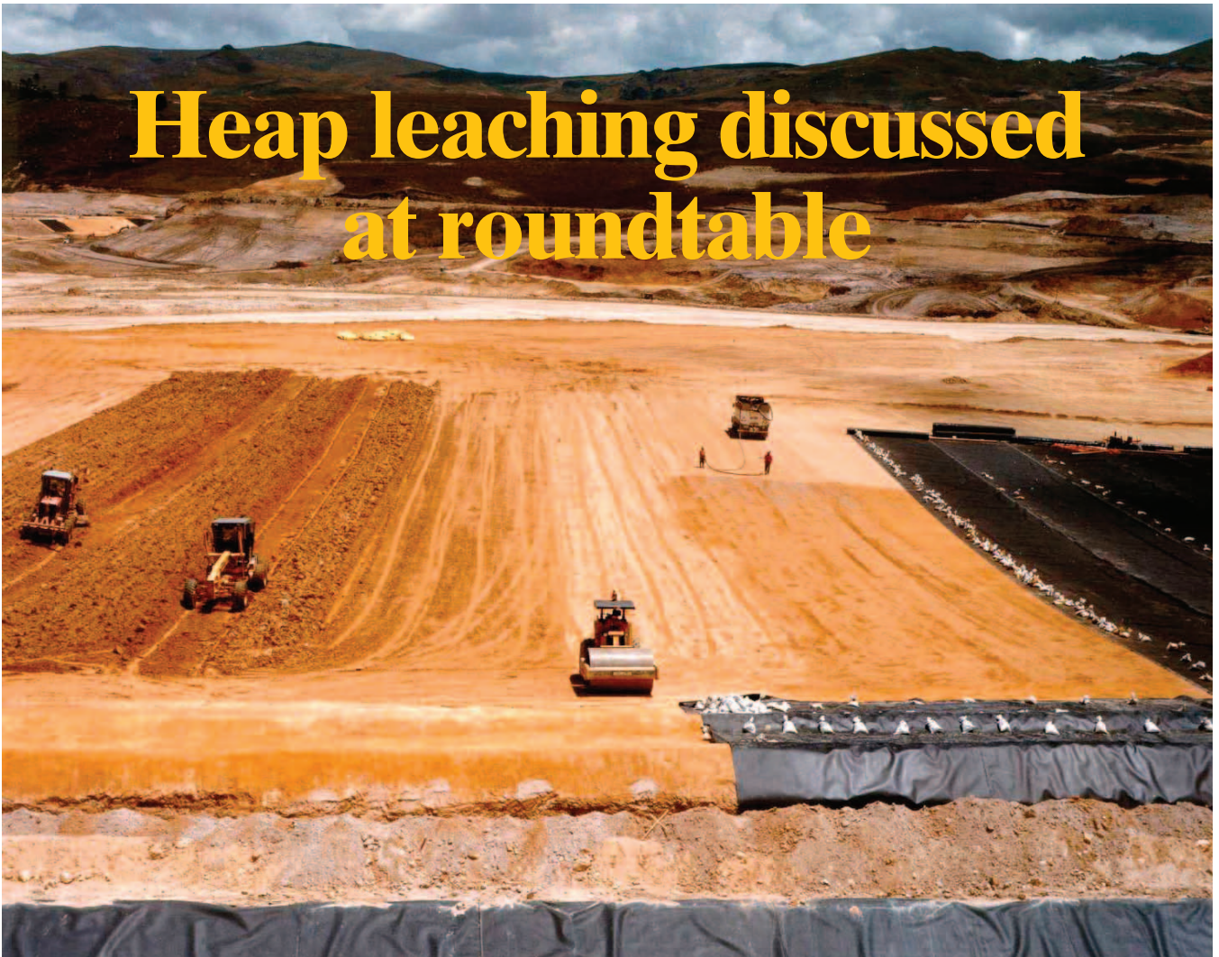
Placement and compaction of a soil liner and the placement of a geomembrane liner at a heap leach operation.
