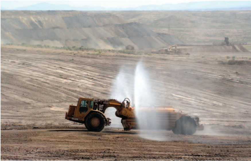
Example of dust suppression and moisture conditioning of soil liner material at a heap leach operation.
