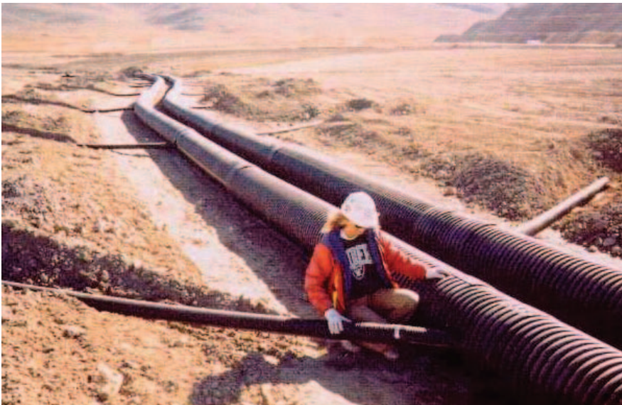
Drainage pipes at the base of a heap leach will assist in the recovery of leachate solutions.
