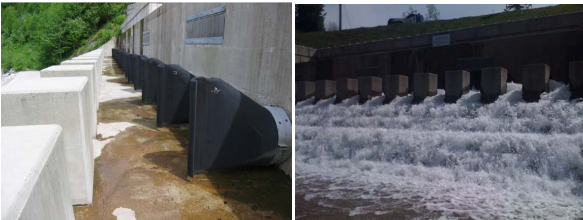
Figure 20: Overflow Spillway with Tideflex valves (left), baffles and steps (right)
