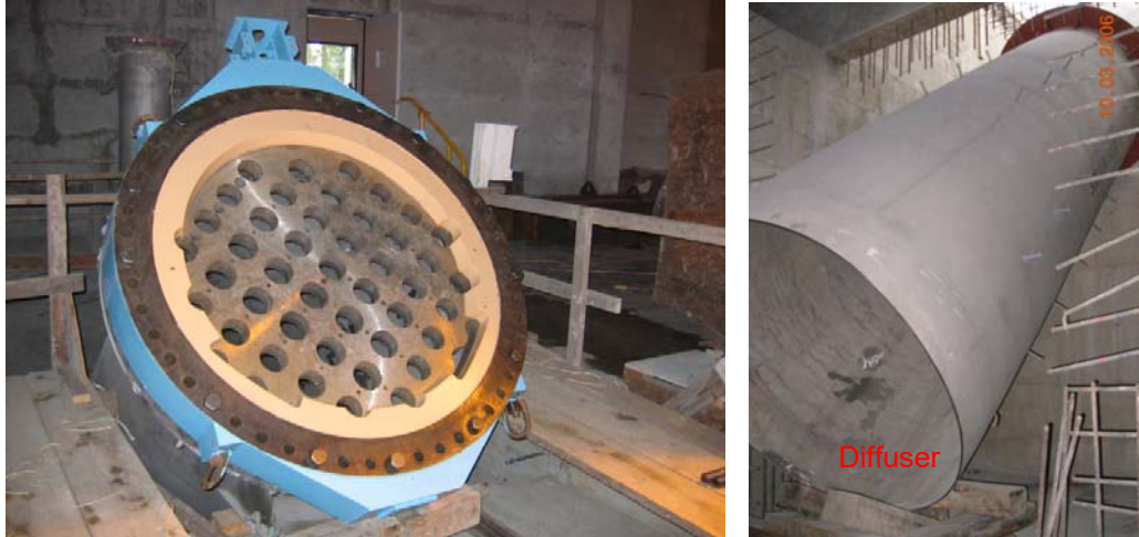
Figure 6: Multi-orifice, sliding plate, energy dissipating PRVs
