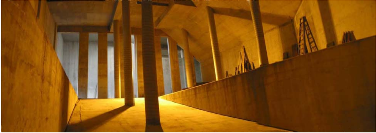
Figure 17: View of interior of Storage Chamber from the bottom of the outlet ramp
