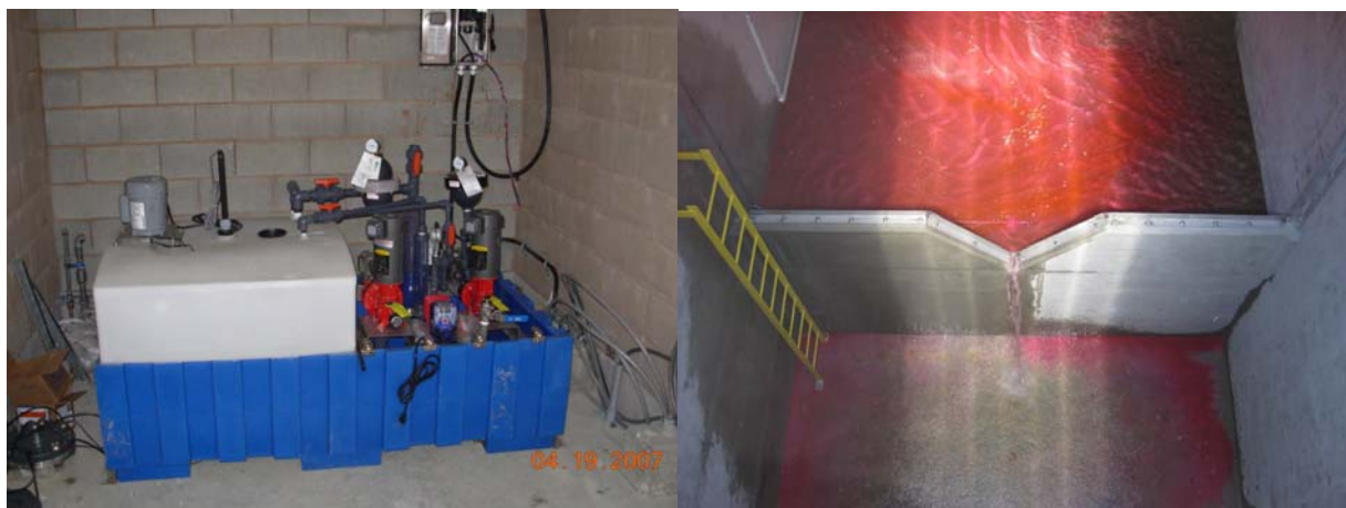
Figure 16: Dechlorination Skid with Tank and Metering Pumps (left). V-notch flow measuring weir in overflow channel (right)
