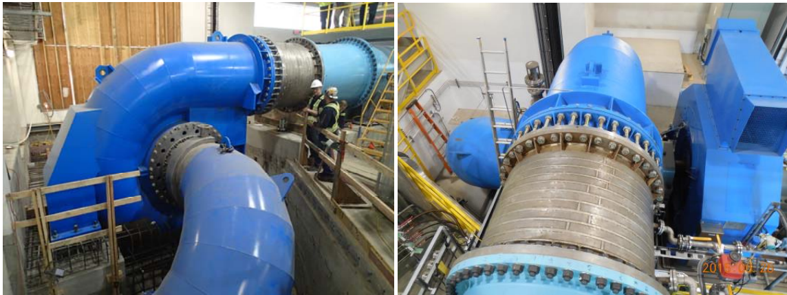
Figure 8: ERF turbine and generator. Note cooling water jacket on turbine inlet pipe.
