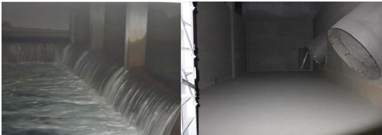
Figure 18: Flow over tailrace weir and PRV discharge weir (left). Interior of discharge chamber showing ends of PRV diffusers (right)
