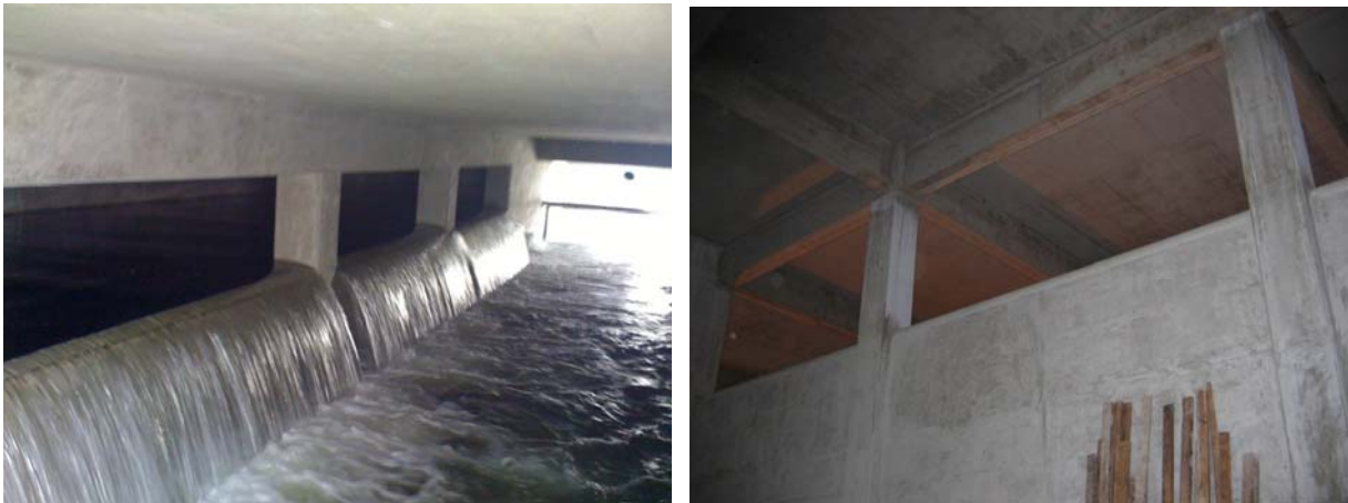
Figure 15: Spill from Tank into overflow channel (left) and view of overflow weir from inside the tank (right)
