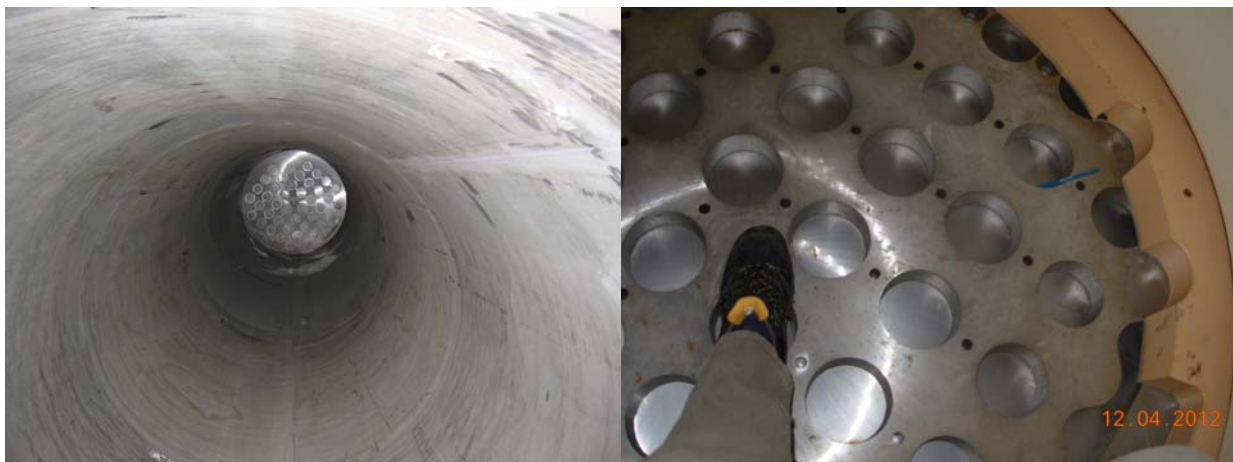
Figure 19: View of MOSPV PRV from downstream end in diffuser (left) and from upstream in piping in Machine Hall (right)
