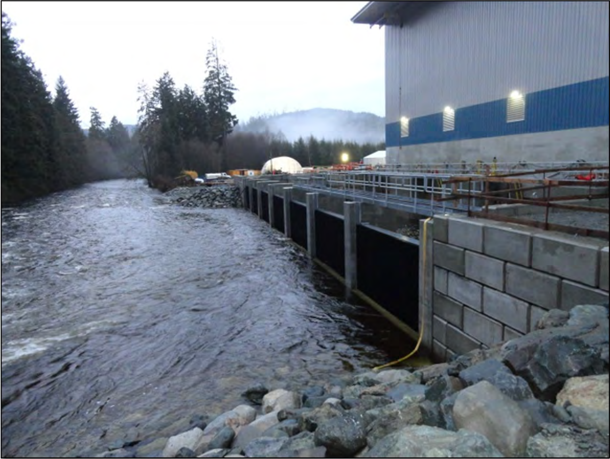
Photo 16 – Fish Screen Fence with Natural Upstream Attraction Flow Visible
