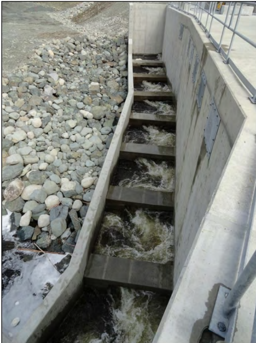
Photo 7 – Fish Ladder Channel in Operation
