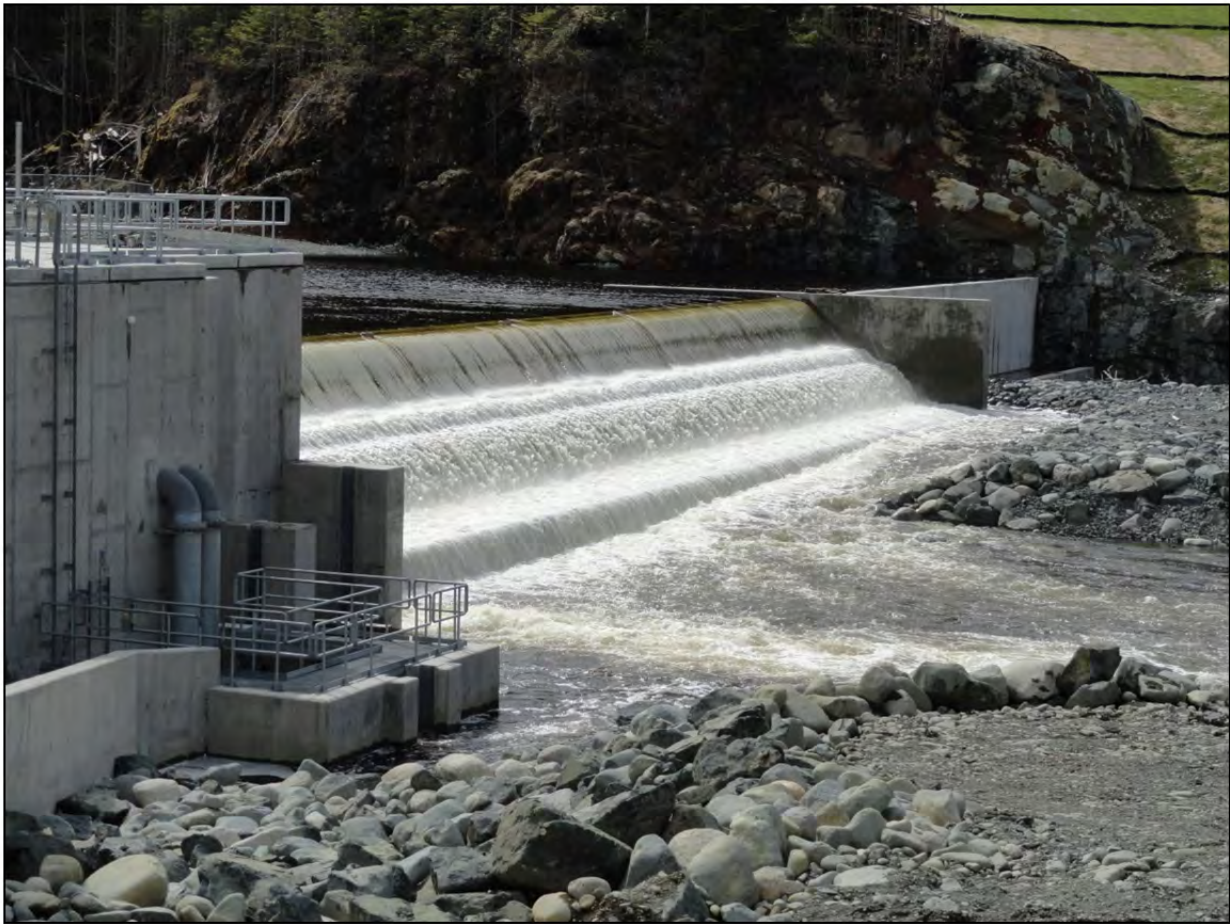
Photo 5 – Diversion Weir with Sluice Channel Outlet and Fish Ladder Entrance on Nearside
