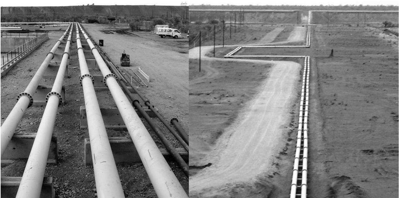
Figure 7 Typical surface tailings pipelines (expansion loop to cater for temperature variation)
