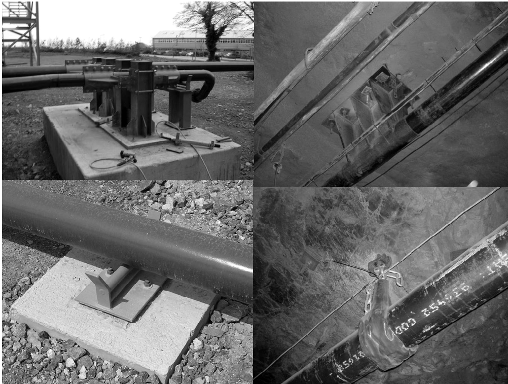
Figure 8 Typical backfill pipe supports (top: anchors, bottom supports; left: surface, right underground)
