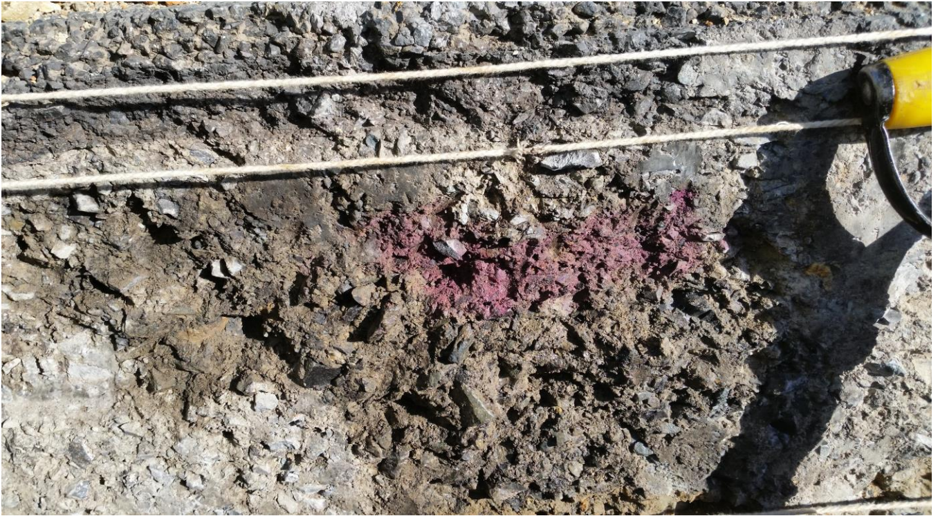
Fig. 3. Typical example of active cement pockets within the BSM layer on the N7
