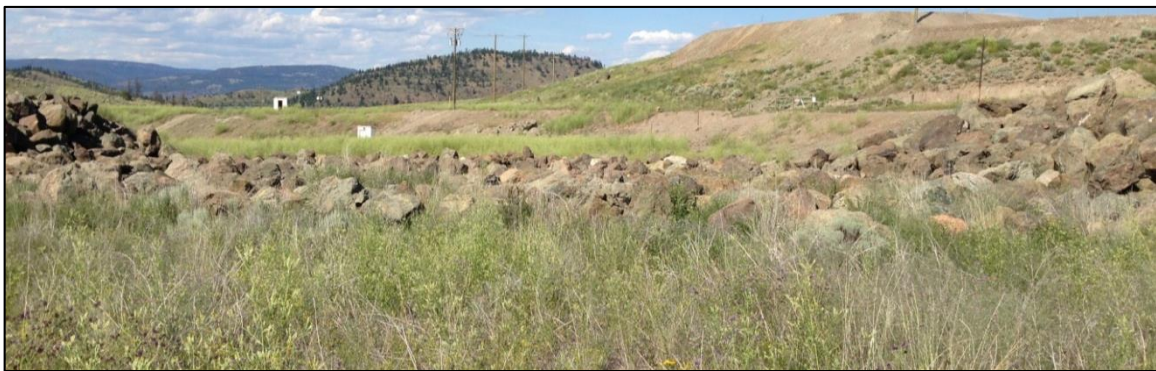
Figure 4: Riprap lined spillway entrance with reclaimed tailings beach in the foreground and mine rock dump on the right side of the frame, looking downstream (northeast)
